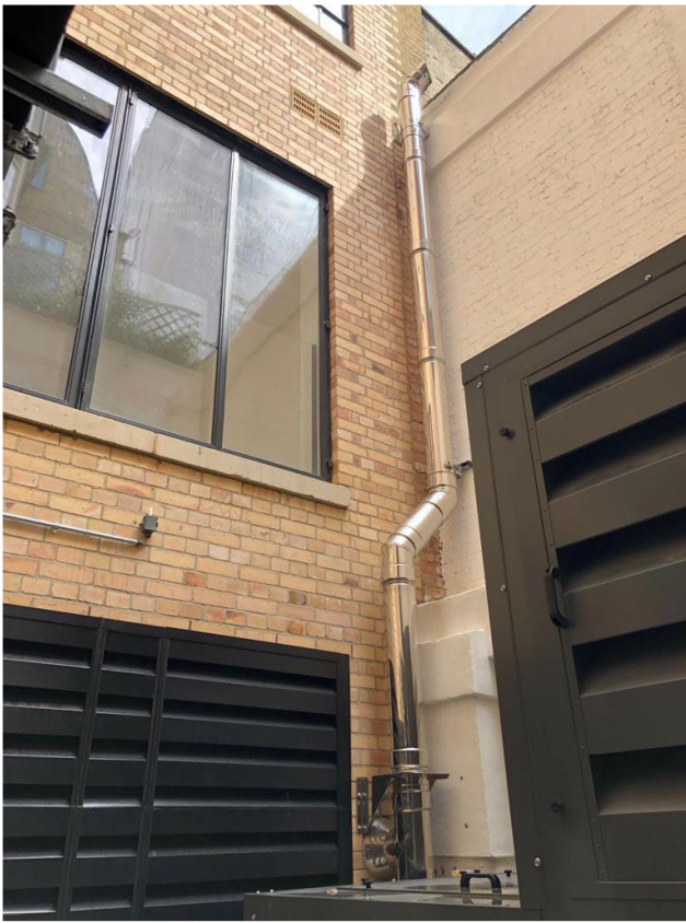
Generator exhaust flue
