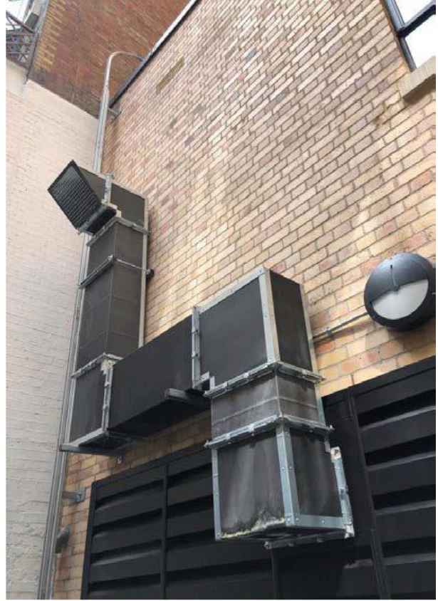
Smoke extract duct
