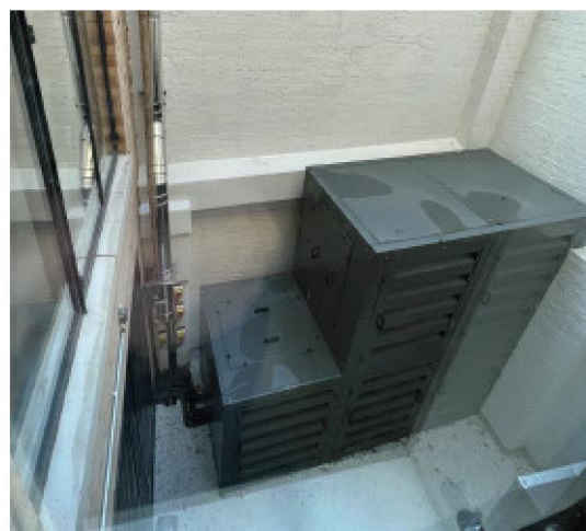
Fig. 14 - View from ground floor unit of installed CU enclosure
